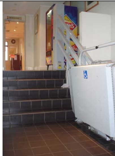
Photo: Stairlift to the restaurant area. Lift is staff operated.
