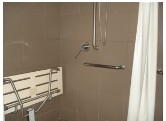
Photo: Shower area with plastic strip on the floor and fold down shower seat.
