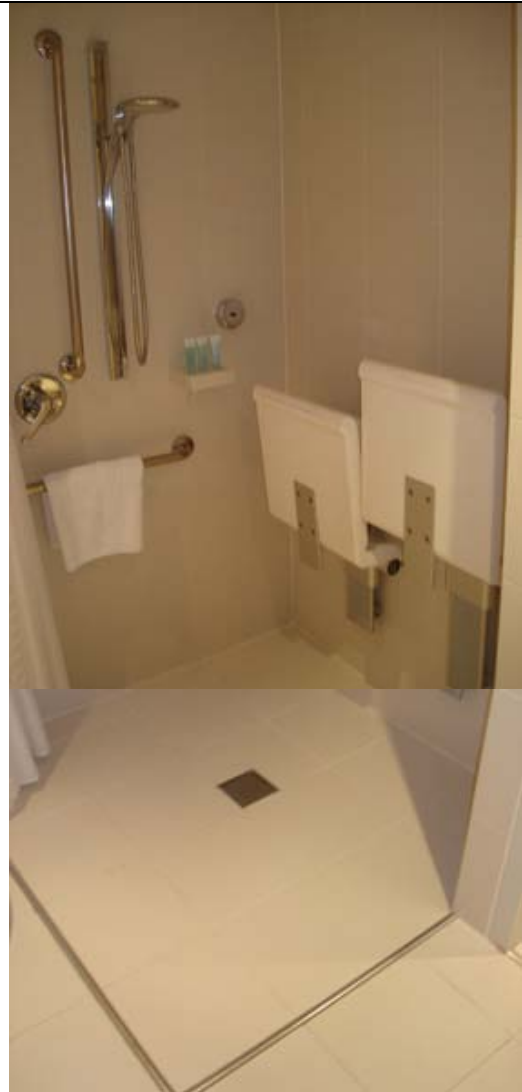
Combined image Photo: Roll-in shower, lever taps and grab rail. Note metal the strip on the floor.
